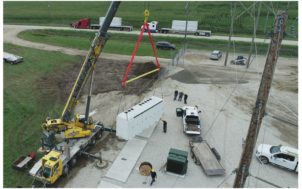
Corn Belt Power recently installed a Tesla® Megapack at their Hampton Substation
